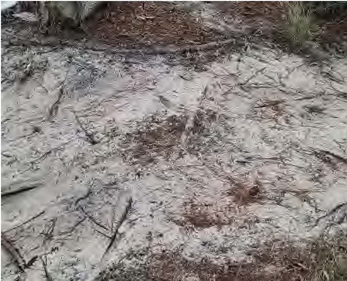
Cut Through #1 Root Damage Berm Top
